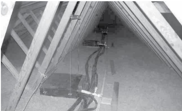
Mounting-Threaded Rod Hung on Truss
