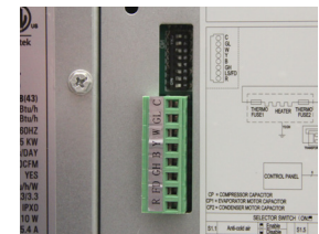
Energy Management & Thermostat Connections
